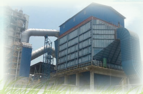
The bag filter system at the 3# kiln front of China Resources Cement (Pingnan) Limited
